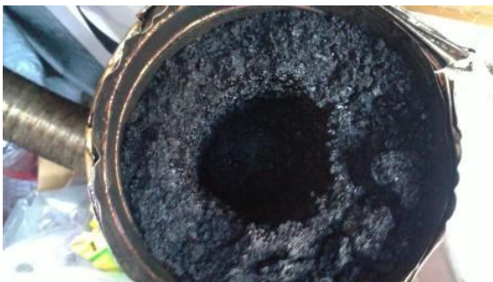
150mm chimney liner blocked with deposits
